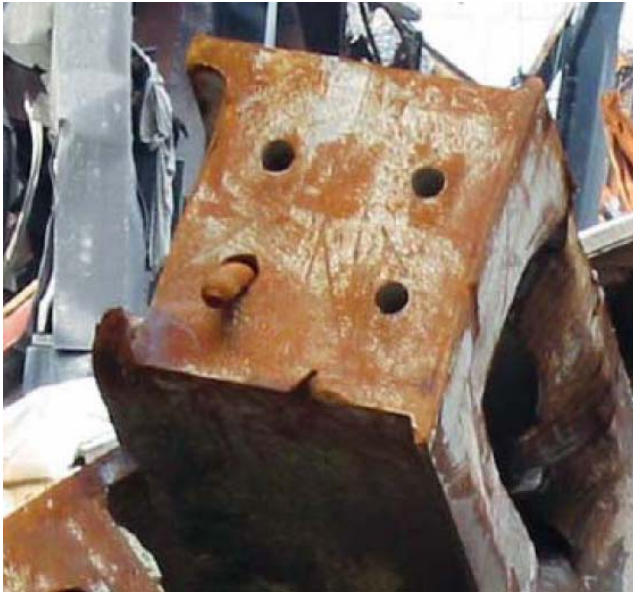
Failed connections in the collapse of WTC buildings
