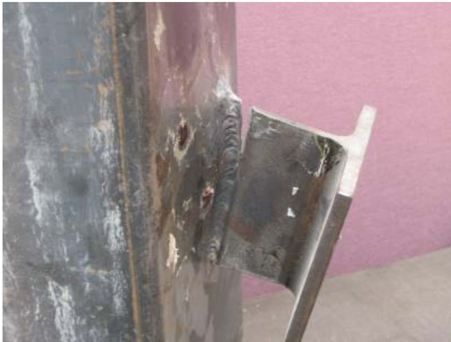
Failure mode (a)
