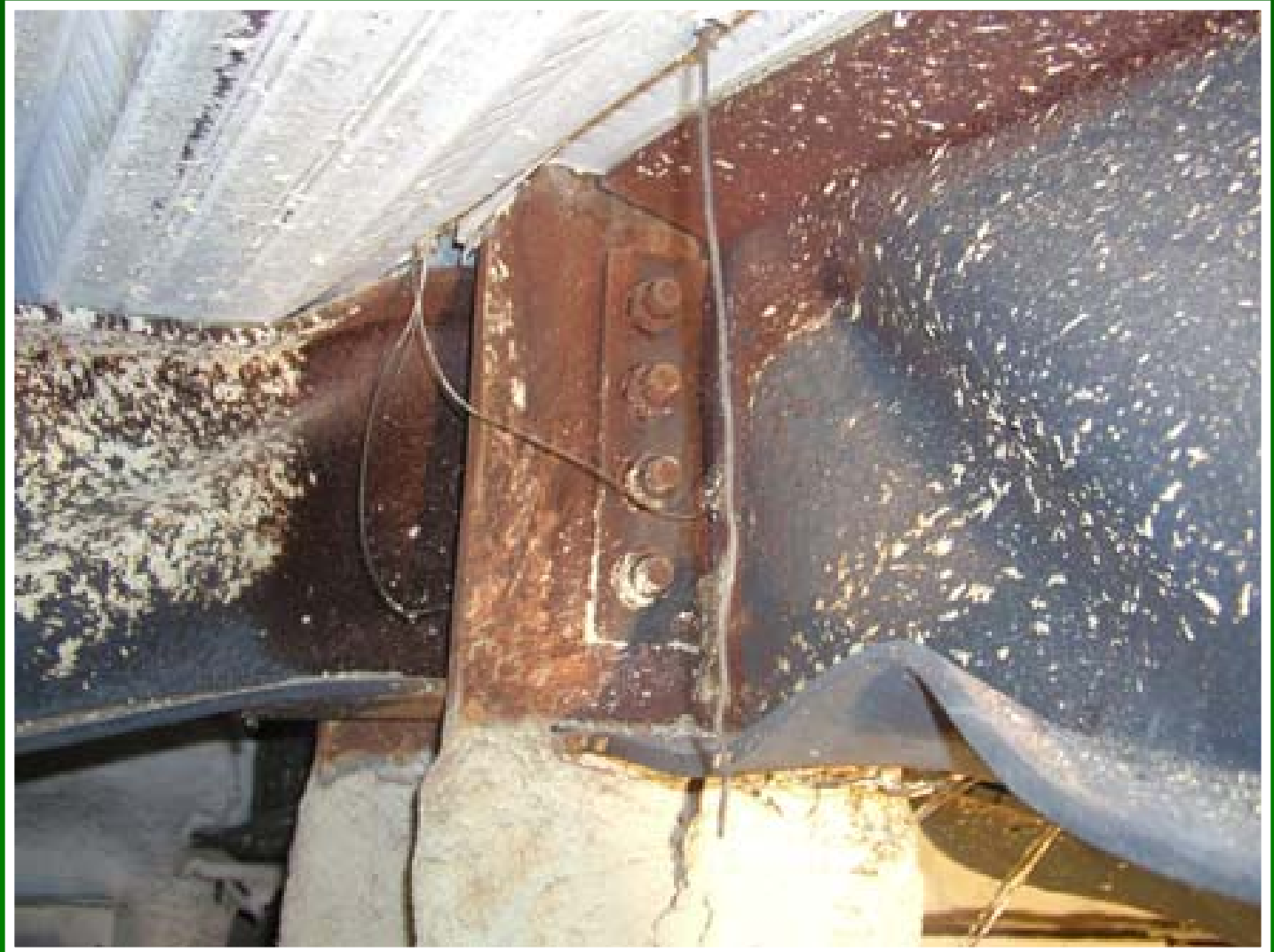
Beam shear buckling
